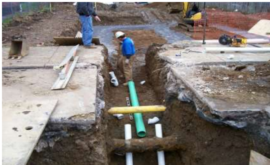
Plumbing Infrastructure Three Bedroom UFAS Compliant Unit
