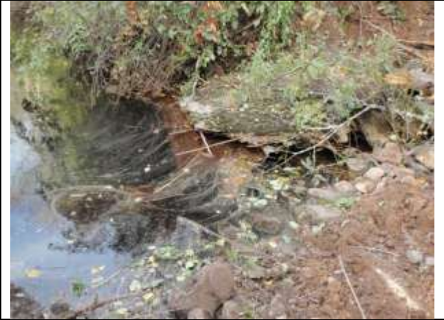
Submerged culvert during high tide.
