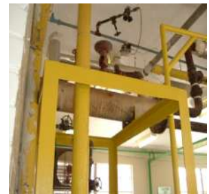
MEP Control Valves
