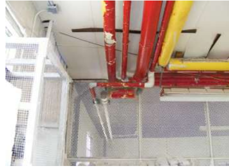
Mechanical and Plumbing Ducting Systems
