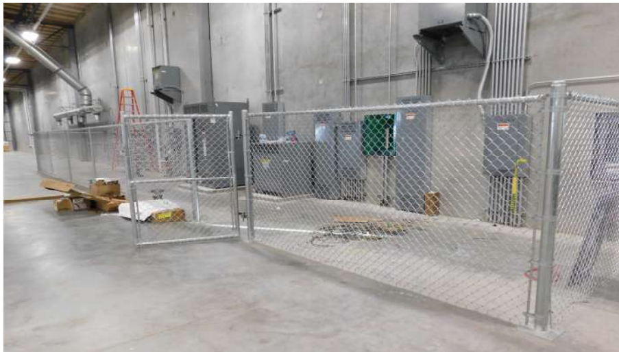
Power Distribution Station Facility Sorting and Distribution Center
