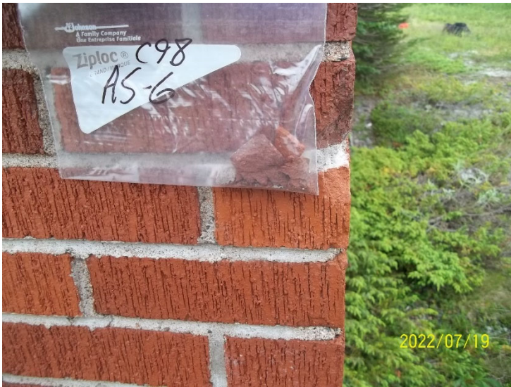
Photo 17: View of bulk material sample C98 AS-6, brick and mortar, cabin exterior.
