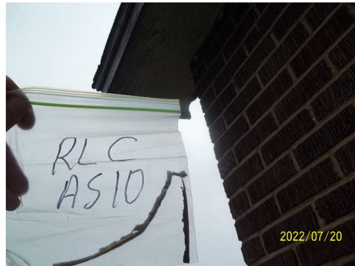
Photo 16: View of bulk material sample RLC AS-10, caulking, cabin exterior.
