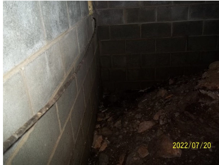
Photo 6: View of the crawl space beneath the accommodations cabin at Rainy Lake Camp.
