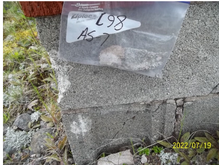
Photo 18: View of bulk material sample C98 AS-7, cinder block and mortar, cabin exterior.
