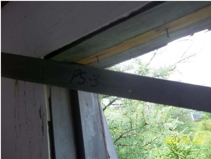
Photo 19: View of paint sample RLC PS-3, wall, outhouse interior.
