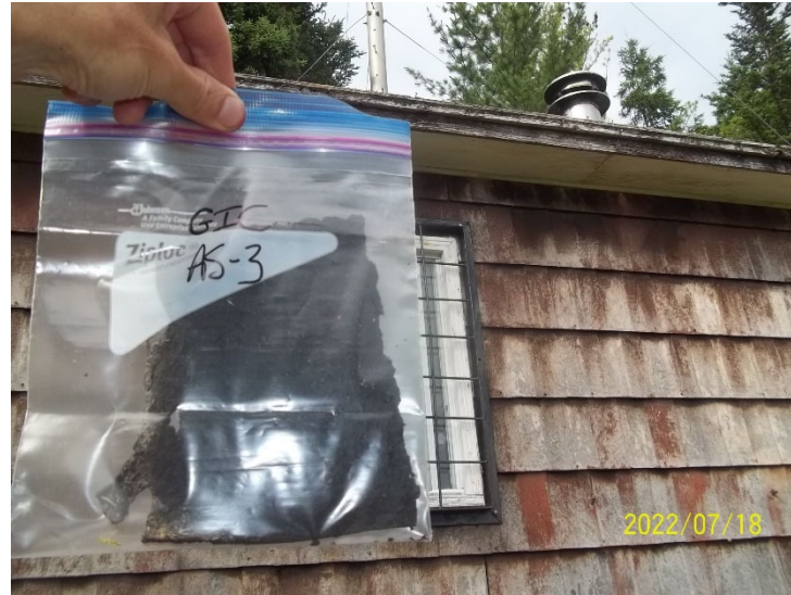
Photo 14: View of bulk material sample GIC AS-3, shingle and flashing, cabin exterior. 40% Chrysotile asbestos.
