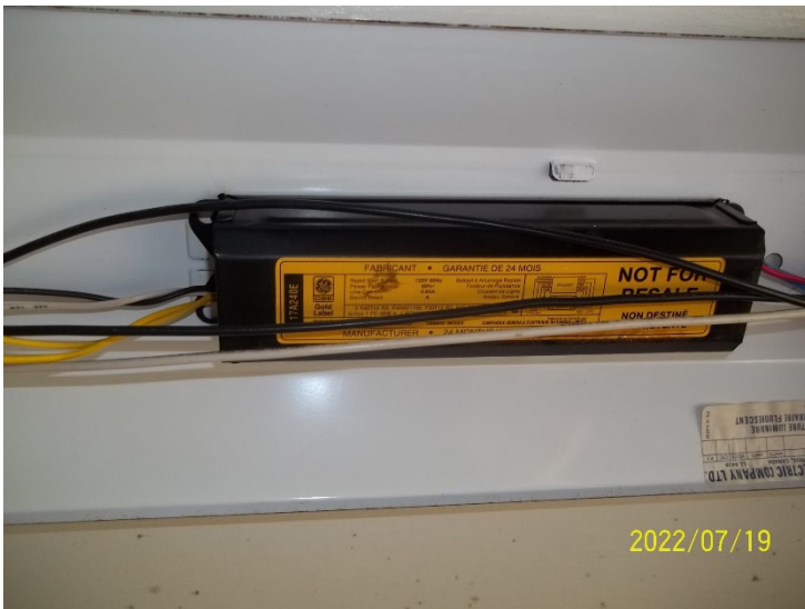
Photo 31: View of fluorescent light ballast inside the accommodations cabin.
