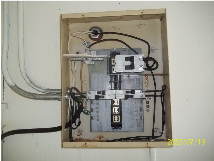
Photo 29: View of electrical panel, cabin interior.
