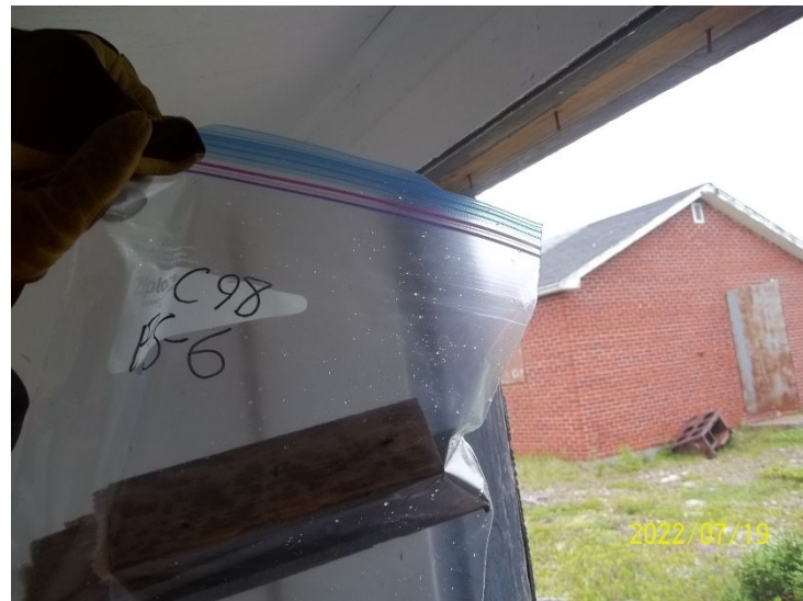
Photo 28: View of paint sample C98 PS-6, wall, outhouse interior.
