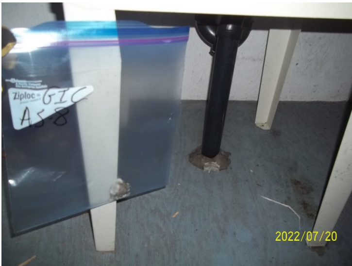
Photo 19: View of bulk material sample GIC AS-8, putty, cabin interior. 9.7% Chrysotile asbestos.
