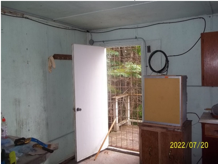
Photo 7: View of the kitchen area inside the accommodations cabin at Glover Island Camp.
