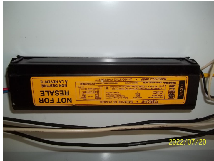
Photo 22: View of fluorescent light ballast, cabin interior.
