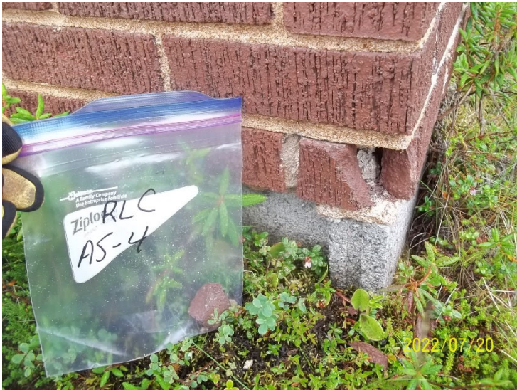
Photo 11: View of bulk material sample RLC AS-4, brick and mortar, cabin interior.
