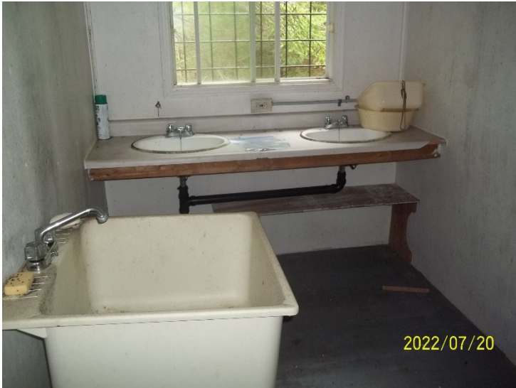
Photo 9: View of the washroom area inside accommodations cabin at Glover Island Camp.
