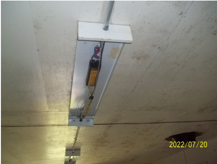
Photo 21: View of fluorescent light fixtures, cabin interior.
