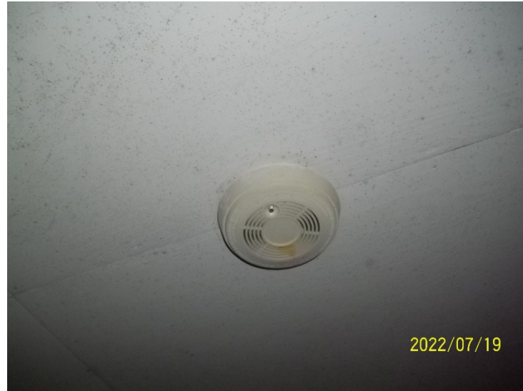
Photo 26: View of smoke detector inside the accomodations cabin.
