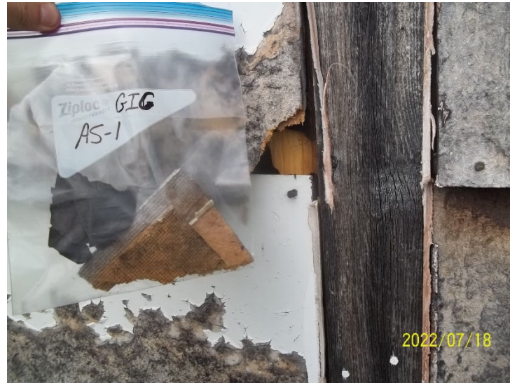
Photo 12: View of bulk material sample GIC AS-1, particle board with tar paper and caulking, cabin exterior.
