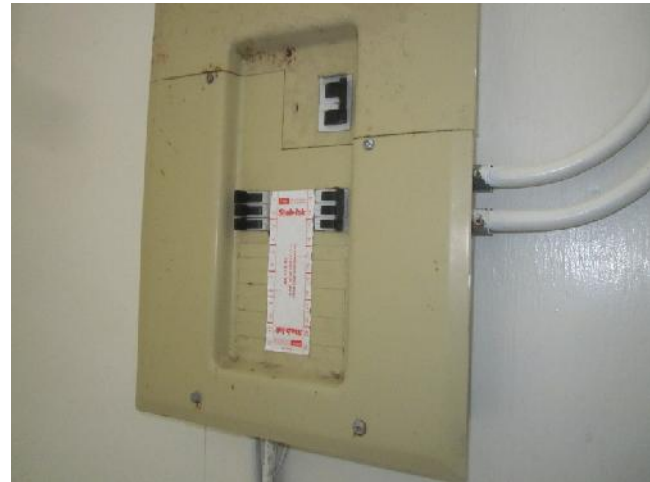
Photo 36: View of electrical panel, cabin interior.
