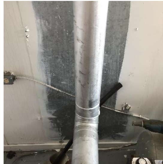
Photo 36: View of ducting from propane stove, cabin interior.
