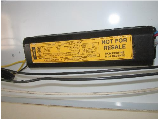
Photo 33: View of fluorescent light ballast, cabin interior.
