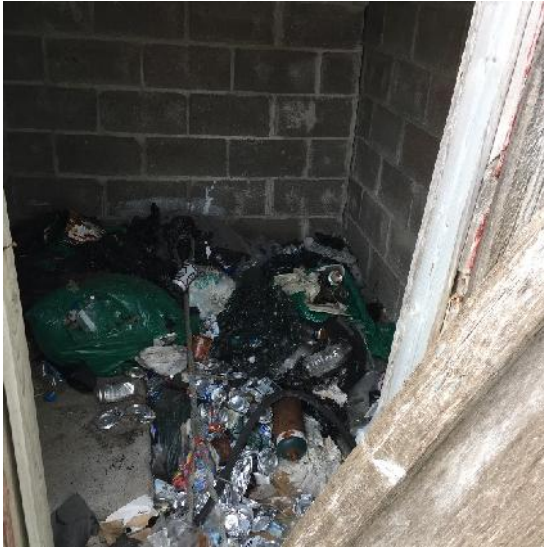
Photo 13: View of interior of the generator shed (attached to the accommodations cabin) at Camp #1.
