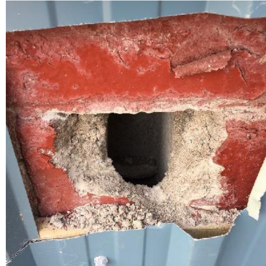
Photo 14: View of cavity inspection location in an exterior wall of the accommodations cabin at Camp #1.
