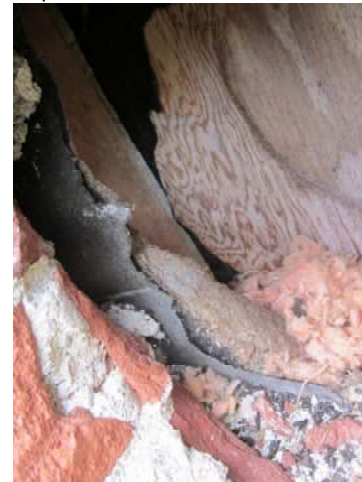
Photo 12: View of cavity inspection in wall from exterior accommodations cabin at Hungry Grove Pond Camp.
