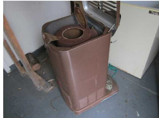
Photo 32: View of oil fired heater, cabin interior.
