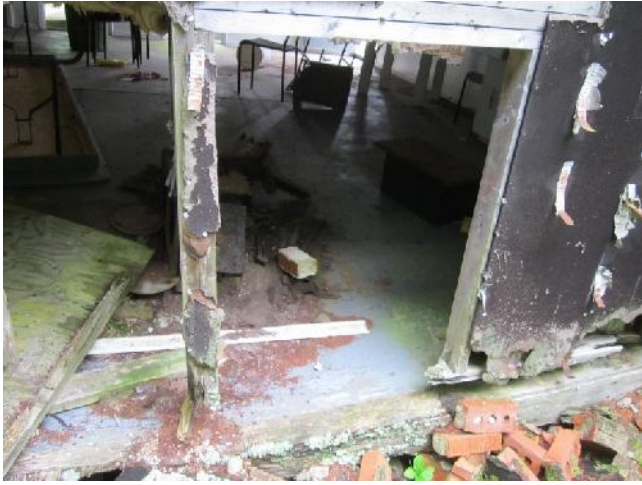
Photo 9: View of collapsed room, on eastern corner of the accommodations cabin.
