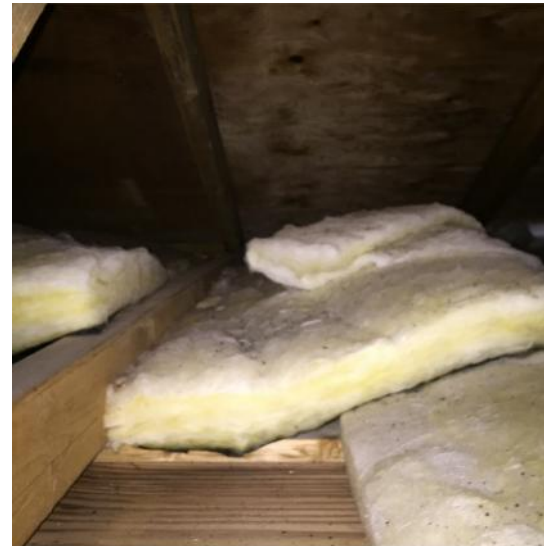
Photo 12: View of the attic inside the accommodations cabin at Camp #1 (Note: attic hatch in the ceiling of Room 1).
