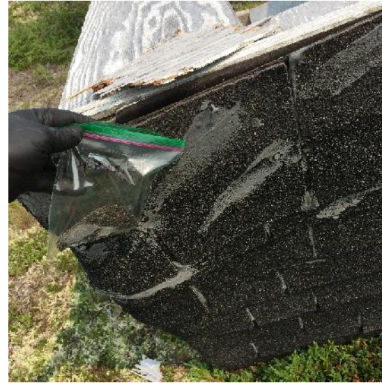
Photo 22: View of bulk material sample PP-PP-AS1, black shingle and tar, outhouse exterior. 1.1 % Cryotile Asbestos
