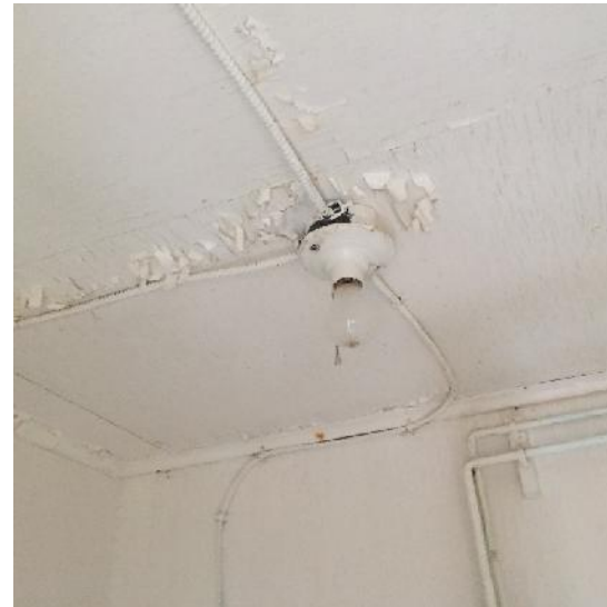
Photo 32: View of incandescent lighting inside accommodations cabin.
