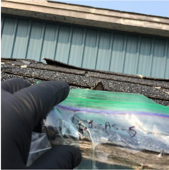
Photo 21: View of bulk material sample C1-AS-5, black shingle and tar, cabin exterior.
