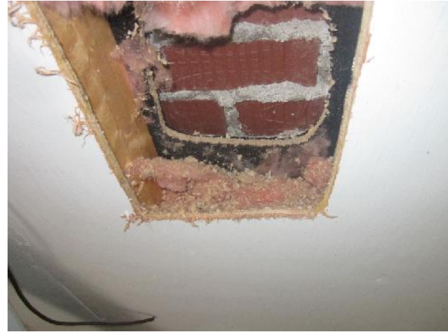
Photo 10: View of the cavity inspection in the interior wall of Room 1 at Mitchell's Pond Camp.
