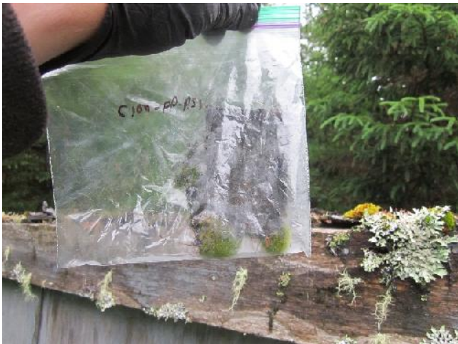
Photo 19: View of bulk material sample C100-PP-AS1, black felt and tar, outhouse exterior. 1.1 % Cryotile Asbestos
