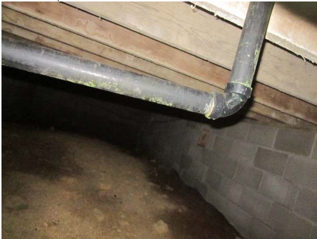
Photo 11: View of cavity inspection below floors in accommodations cabin at Hungry Grove Pond Camp.
