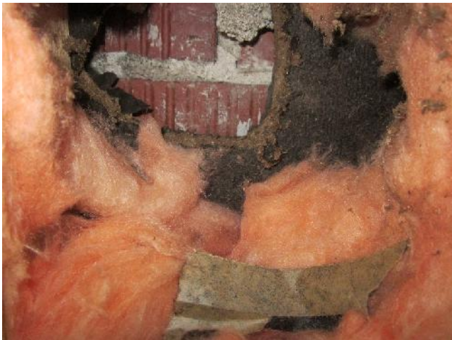
Photo 11: View of cavity inspection in wall of accommodations cabin at Medonnegonik Camp.
