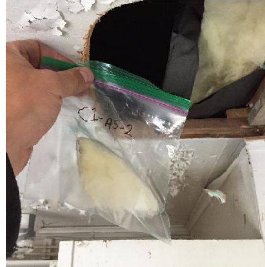
Photo 18: View of bulk material sample C1-AS-2, black paper backing and yellow fibreglass insulation, cabin interior.
