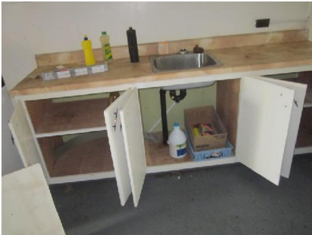
Photo 35: View of kitchen sink plumbing, cabin interior.
