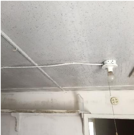
Photo 35: View of incandescent lighting and smoke detector, cabin interior.
