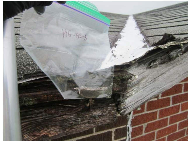
Photo 20: View of bulk material sample HG-AS8, black caulking, cabin exterior.
