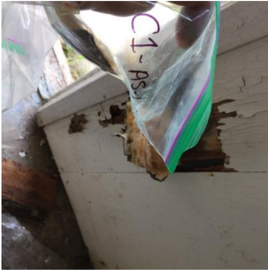
Photo 17: View of bulk material sample C1-AS-1, black paper backing and pink fibreglass insulation, cabin interior.
