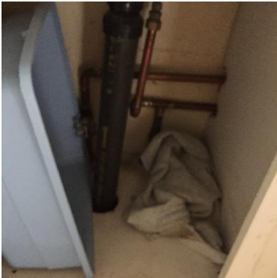
Photo 35: View of copper piping under the sink in kitchen of the accomodations cabin.
