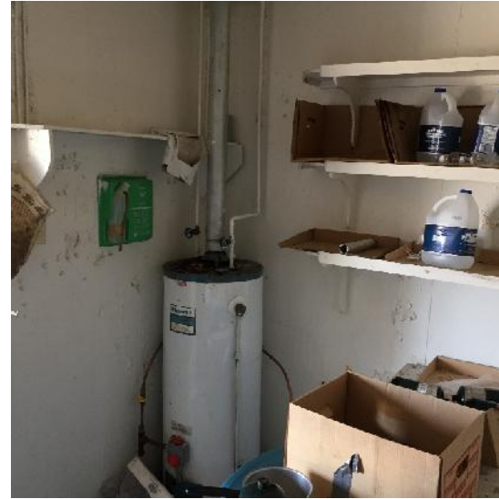
Photo 34: View of propane hot water tank inside the accomodations cabin.
