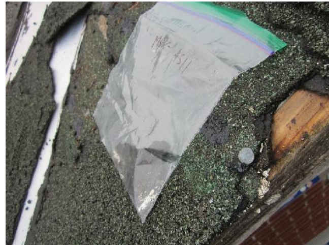
Photo 24: View of bulk material sample MDX-AS11, green/black shingle and tar, cabin exterior.
