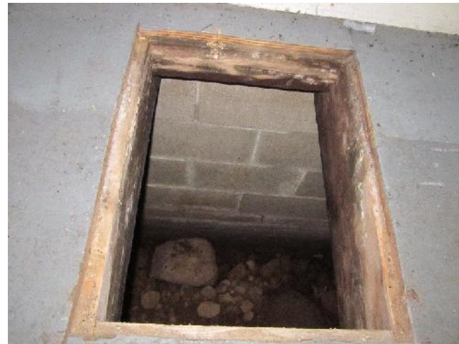
Photo 12: View of cavity inspection in the floor of the accommodations cabin at Medonnegonik Camp.
