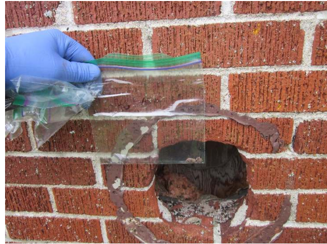
Photo 22: View of bulk material sample HG-AS10, red sealant, cabin exterior.
