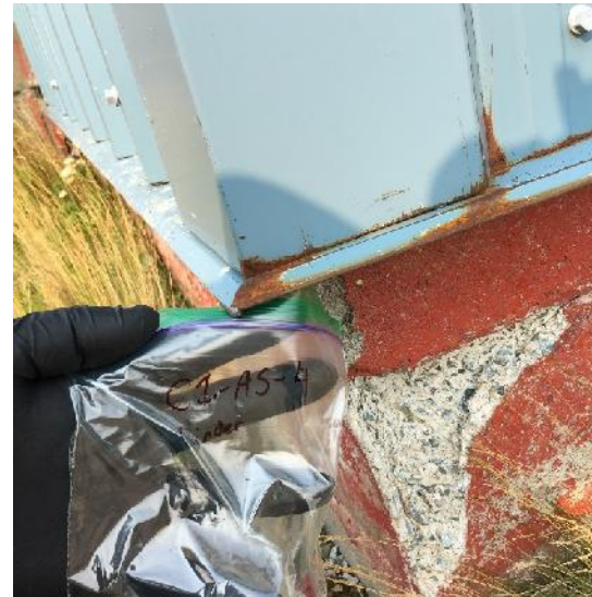
Photo 20: View of bulk material sample C1-AS-4, concrete block and mortar, cabin exterior.
