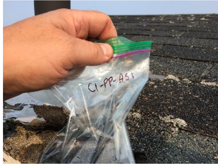
Photo 22: View of bulk material sample C1-PP-AS1, black shingle and tar, outhouse exterior.
