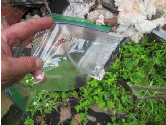
Photo 17: View of bulk material sample C100-AS-5, black tar, cabin exterior. 21.2 % Cryotile Asbestos
