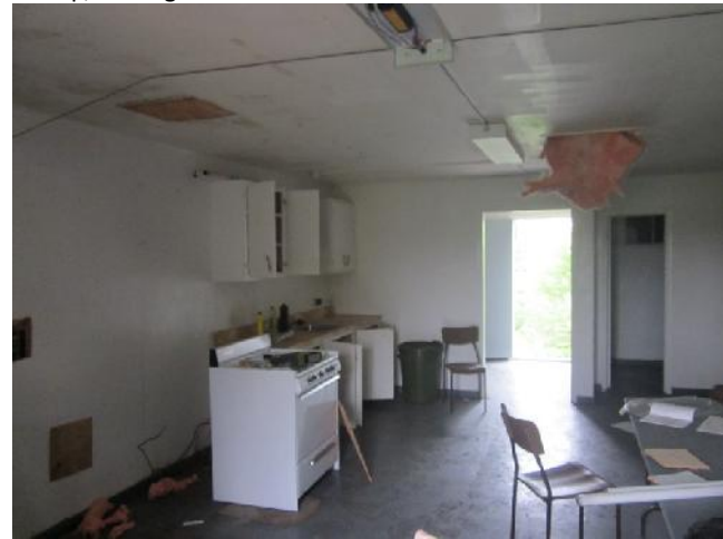
Photo 4: View of the kitchen area of the accommodations cabin at Mitchell's Pond Camp.
