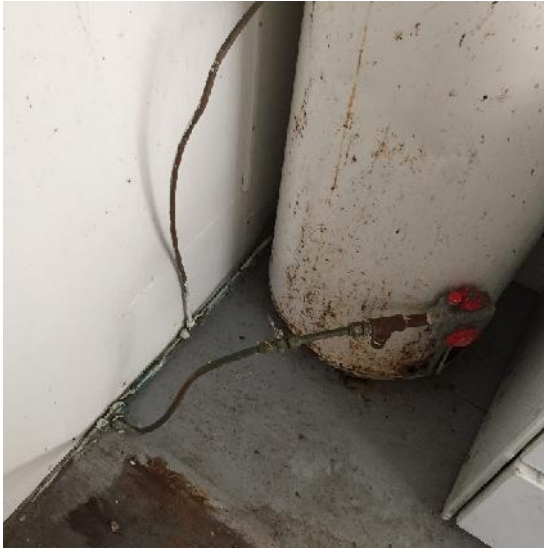
Photo 33: View of propane fired hot water tank and copper pipes, cabin interior.
