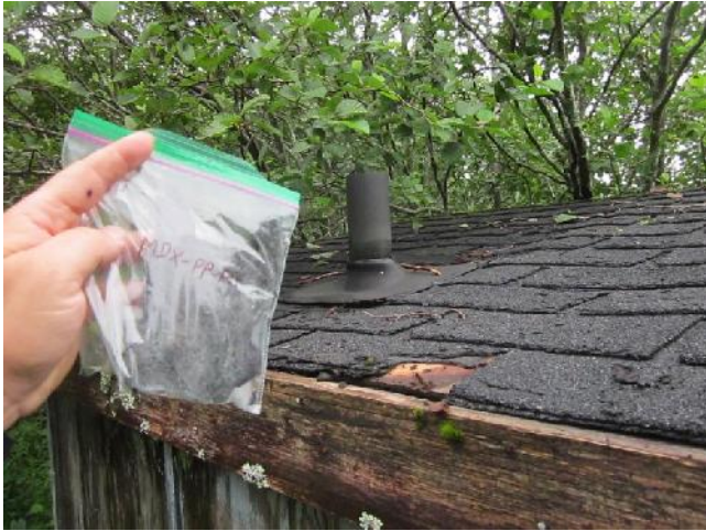
Photo 25: View of bulk material sample MDX-PP-AS1, black shingle and tar, outhouse exterior.
