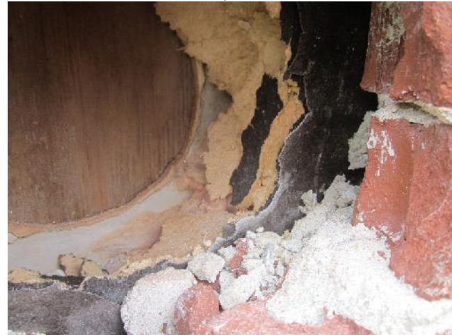
Photo 12: View of cavity inspection in the wall of the exterior of the accommodations cabin at Mitchell's Pond Camp.
