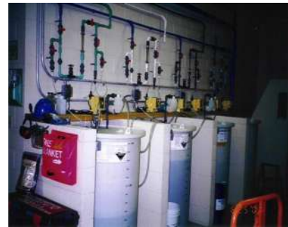
Chemical Feed Room
