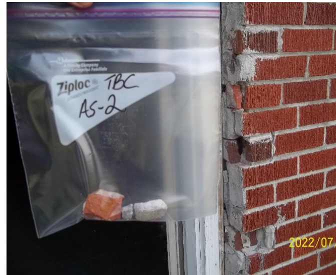
Photo 14: View of bulk material sample TBC AS-2, brick and mortar, cabin exterior.
