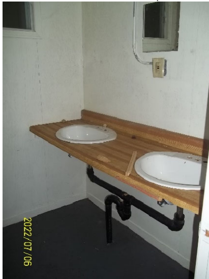
Photo 7: View of the washroom inside the accommodations cabin at Pot Hill Camp.
