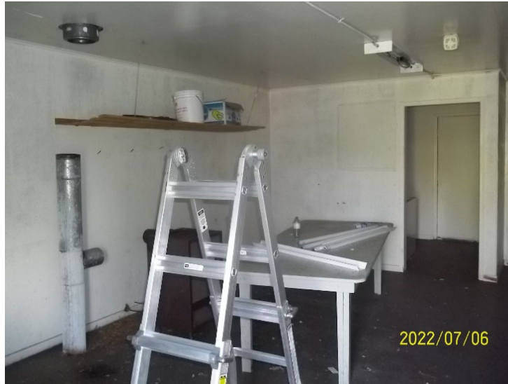
Photo 5: View of the dining area of the accommodations cabin at Three Brooks Camp.
