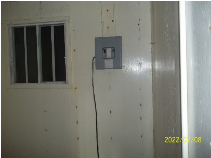
Photo 31: View of electrical panel, cabin interior.
