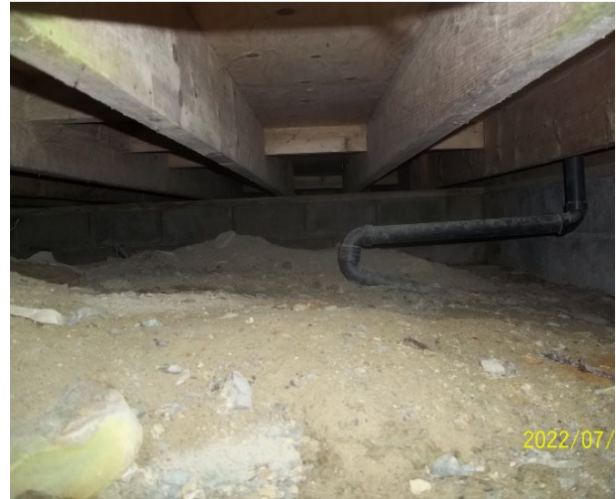
Photo 10: View of the crawl space beneath the accommodations cabin at Three Brooks Camp .
