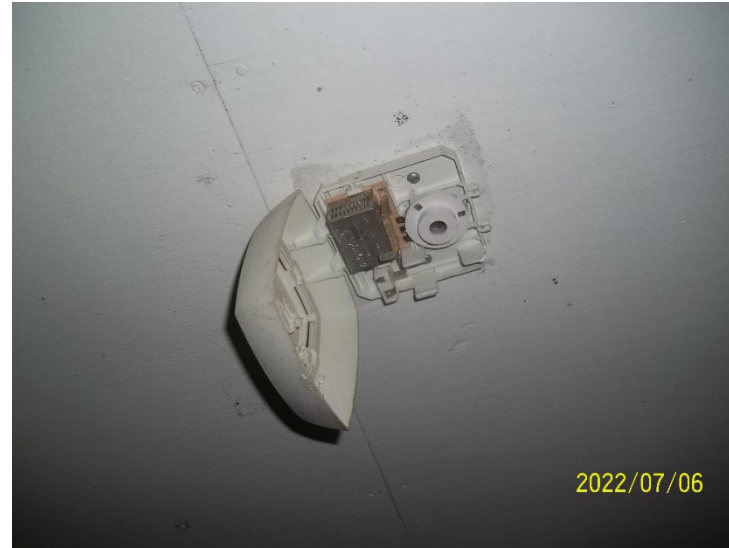
Photo 26: View of smoke detector, cabin interior.
