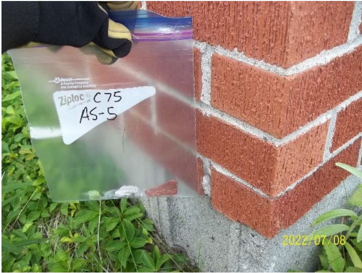
Photo 17: View of bulk material sample C75 AS-5, brick and mortar, cabin exterior.
