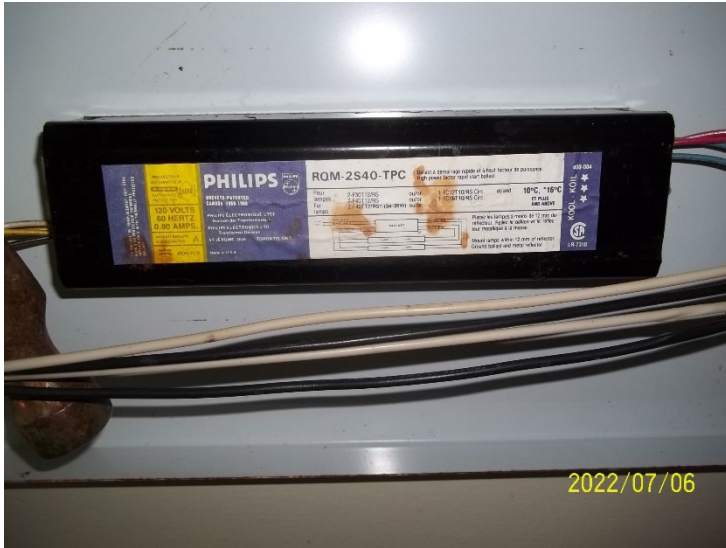
Photo 29: View of fluorescent light ballast. Note: label indicating no PCBs.
