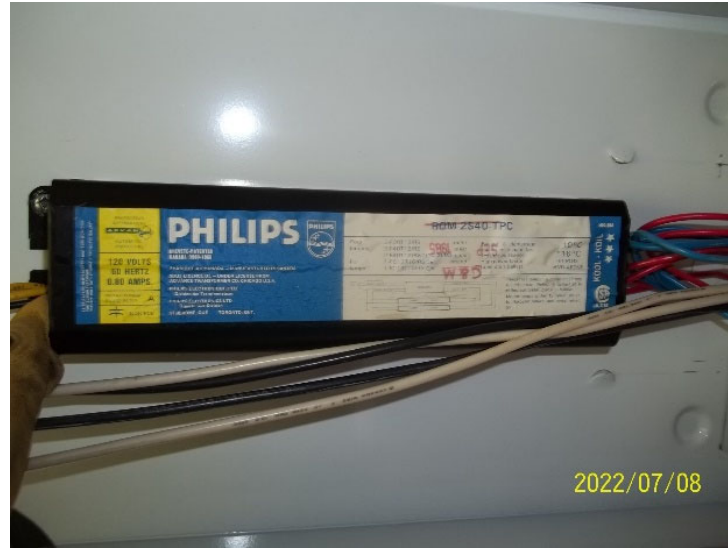
Photo 30: View of fluorescent light ballast. Note: label indicating no PCBs.
