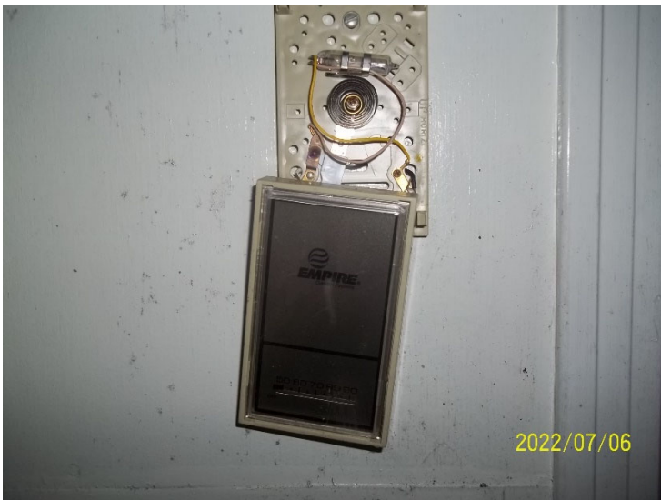
Photo 23: View of mercury-containing thermostat, cabin interior.
