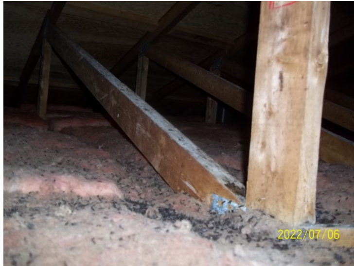
Photo 9: View of the attic in the accommodations cabin at Three Brooks Camp. Note: rodent feces on insulation.
