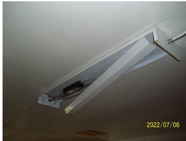
Photo 24: View of fluorescent light fixture, cabin interior.
