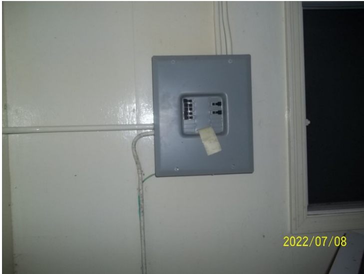
Photo 29: View of electrical panel inside cabin.
