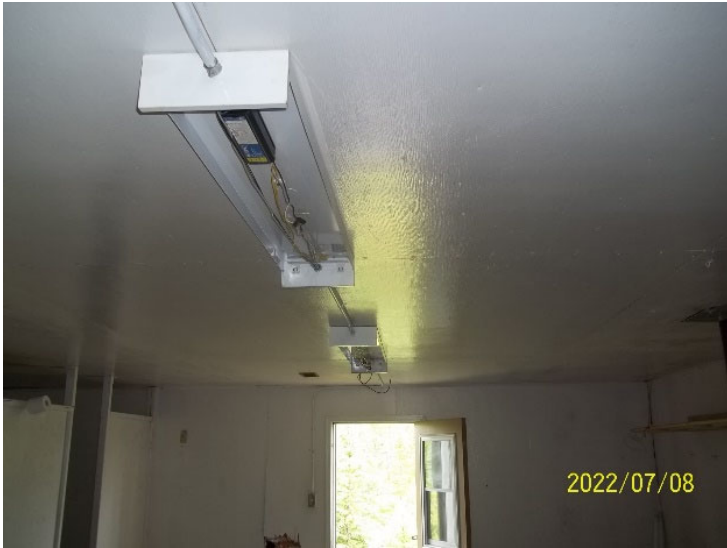
Photo 29: View of fluorescent light fixtures in cabin.
