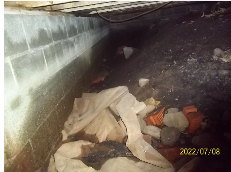
Photo 10: View of the crawl space beneath the accomodations cabin at North West Gander River Camp.
