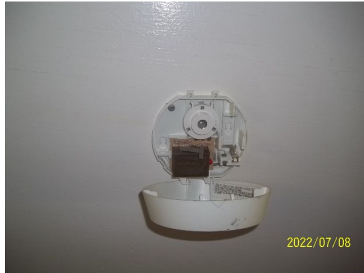
Photo 32: View of smoke detector inside the accommodations cabin.
