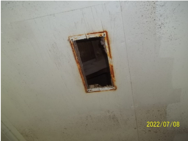
Photo 33: View of suspected mould on ceiling, cabin interior.
