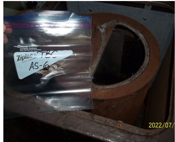
Photo 18: View of bulk material sample TBC AS-6, gasket, cabin interior. 70% Crysofile Asbestos
