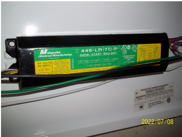
Photo 31: View of fluorescent light ballast. Note: label indicating no PCBs.
