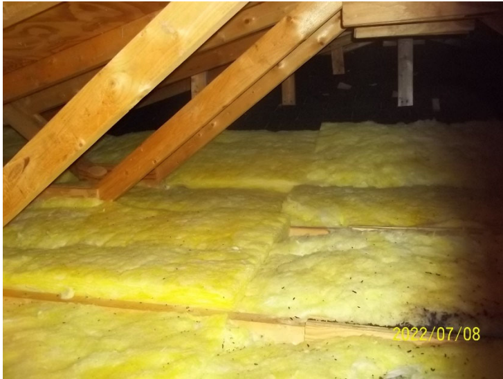
Photo 9: View of the attic in the accomodations cabin at North West Gander River Camp. Note: rodent feces.
