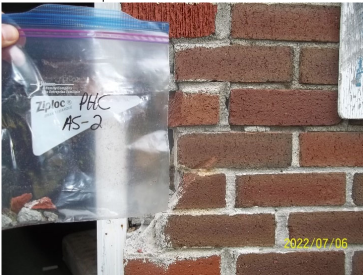
Photo 11: View of bulk material sample PHC AS-2, brick and mortar, cabin exterior.
