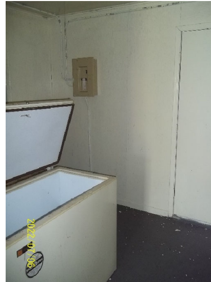
Photo 30: View of freezer and electrical panel, cabin interior.
