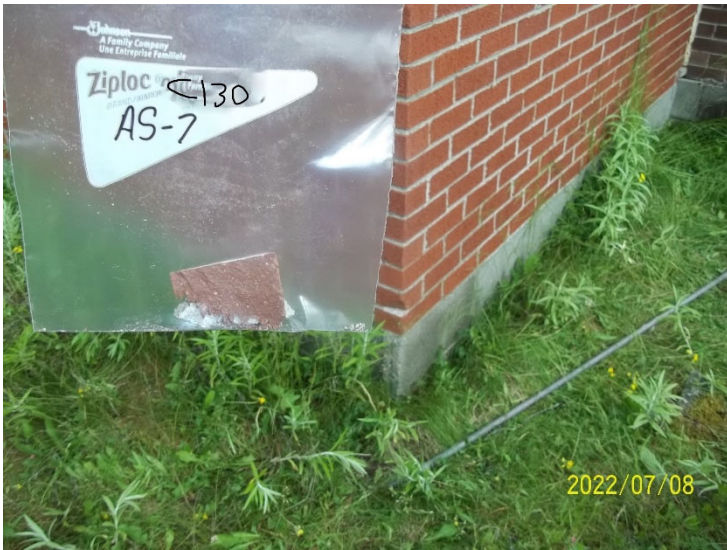
Photo 21: View of bulk material sample C130 AS-7, brick and mortar, cabin exterior.
