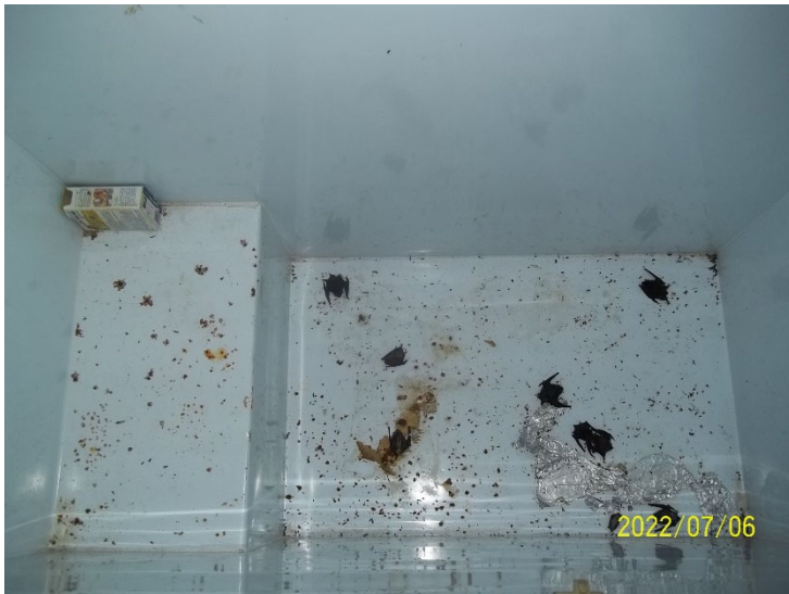
Photo 31: View of dead bats and feces inside the freezer, cabin interior.
